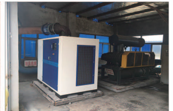
Jiangsu Xuzhou paper plant
