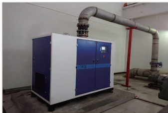
Shunde Ronggui WWTP
