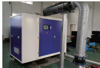
Nanhai Yanbu WWTP
