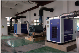
Shanghai Xujing WWTP
